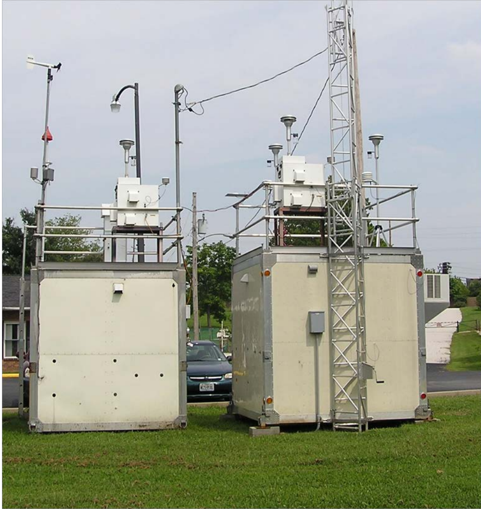
Figure 4. Photograph showing air conditioned monitoring sheds used to house an Xact FLM in Herculaneum, MO.
