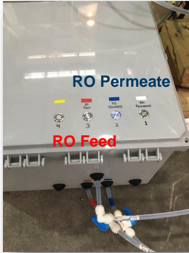
Automated Feed Manifold
