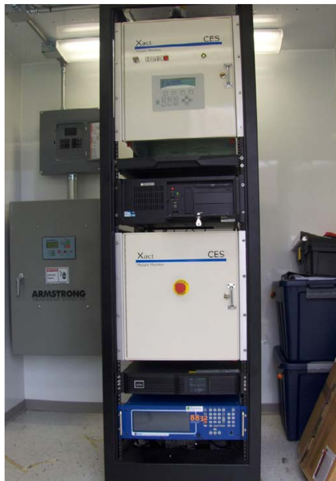
Figure 2-1. Xact 625 installed in field trailer for testing; top to bottom are the control panel/X-ray source, computer, XRF analysis module with sampling tape drive, modem, and datalogger.
